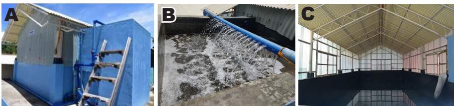
Figure 15. The covered reservoir (A), the sand filter box (B), and the reservoir tank (C)
