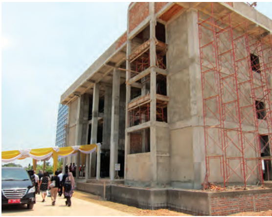
After the signing ceremony and with Prof. Widjaja leading, the SEAFDEC Secretary-General, senior officials of SEAFDEC and delegates from the Member Countries, and the representative of the Governor of South Sumatra visited the construction site of the IFRDMD premises and facilities
