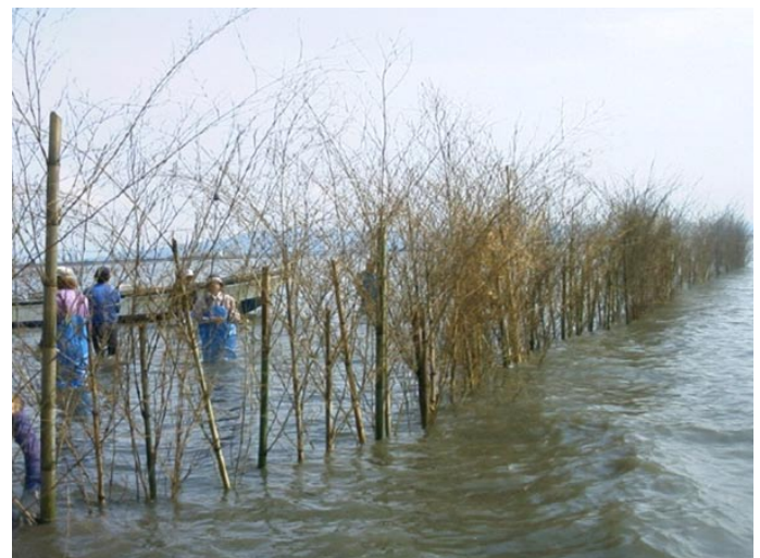
Fig. 10a. Bamboo fence installed to promote settlement of drifting larva (Source: Kumamoto City and Matsuo Fishery Cooperative)
