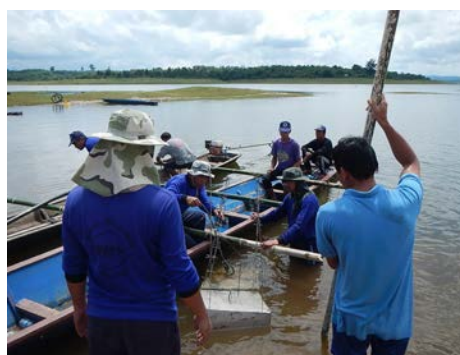
Demonstration and hands-on training for local fisheries officers and fishing community on construction and installation of artificial fish shelters in the conservation area in Nam Houm Reservoir, Lao PDR
