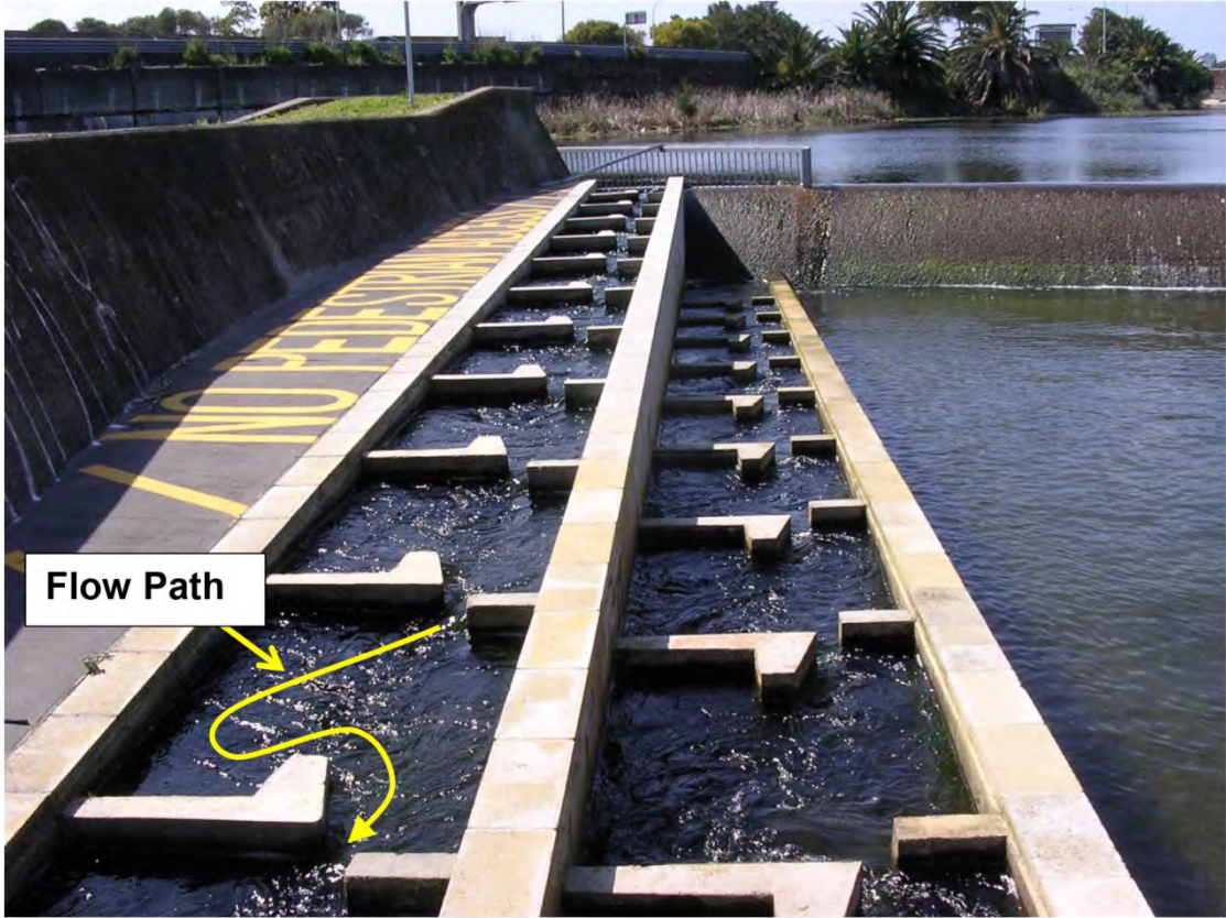
Figure 6. A vertical-slot fishway
