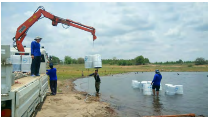
Fig. 5. Installation of buoys to mark the area of the conservation zone and the border between Ban Dong Khampho and Ban Nachuak in Nam Oon Dam
