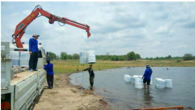
Fig. 5. Installation of buoys to mark the area of the conservation zone and the border between Ban Dong Khampho and Ban Nachuak in Nam Oon Dam
