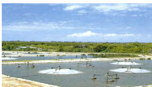
Figure 13. New type of aerator with in-jet system installed under water in ponds
