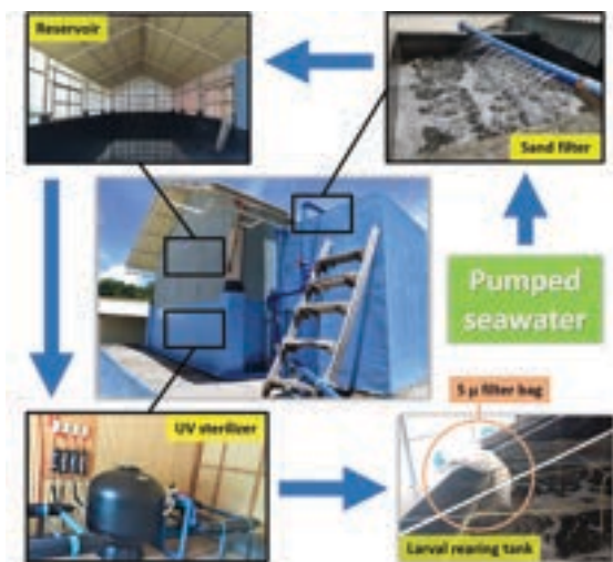
Figure 6. Water filtration and UV sterilization systems at the Shrimp Hatchery Complex of SEAFDEC/AQD
