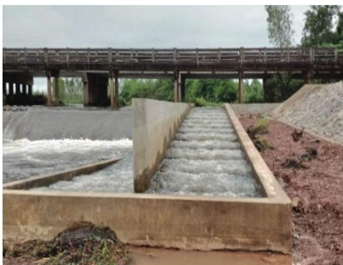
Figure 8. Hauy Wang Chang Weir in Hauy Lung River, Udonthani Province, Thailand (above) and the installed demonstration fish passage (below)
