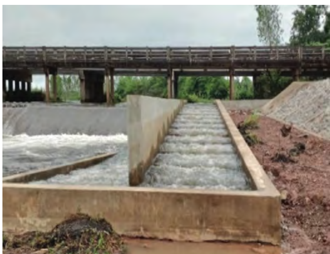
Figure 8. Haiy Wang Chang Weir in Haiy Lung River, Udonthani Province, Thailand (above) and the installed demonstration fish passage (below)
