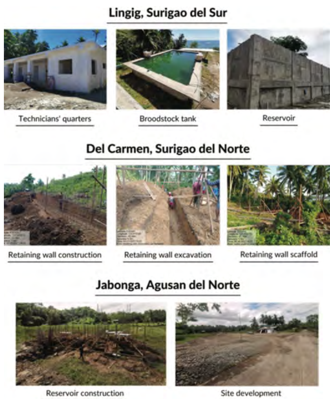
Figure 5. Progress of the construction of the hatcheries in three sites: Lingig (Surigao del Sur), Del Carmen (Surigao del Norte), and Jabonga (Agusan del Norte)
