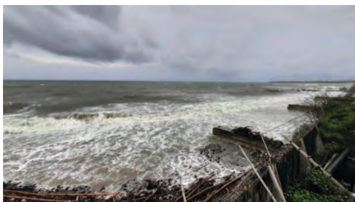
Storm surge threatening the sea wall of AQD's Tigbauan Main Station in Iloilo, Philippines
