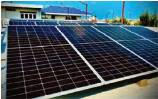
Figure 2. Solar panels installed on the rooftop of one of the SEAFDEC/TD office buildings in 2022
