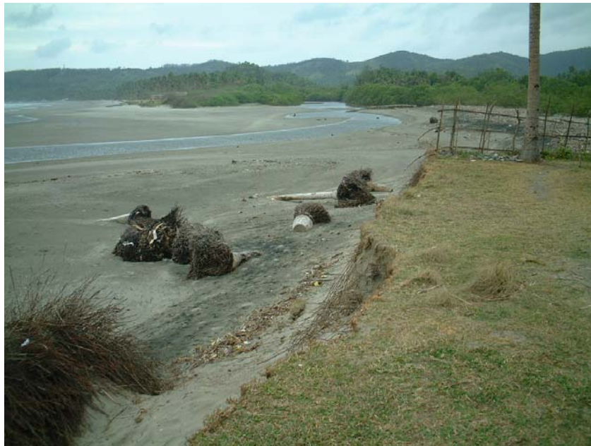
Without its protective mangrove belt, the coast is open typhoons, storm surges, or to riverbank erosion such as here in Aklan, Philippines
