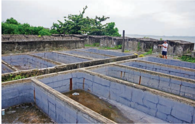
A hatchery in Batan, Aklan which is subjected for repair and rehabilitation courtesy of SEAFDEC/AQD, BFAR-6, and the private sector
