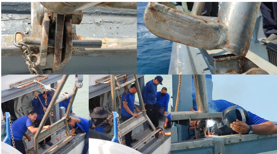
Figure 9. Broken gallow position and reparation
